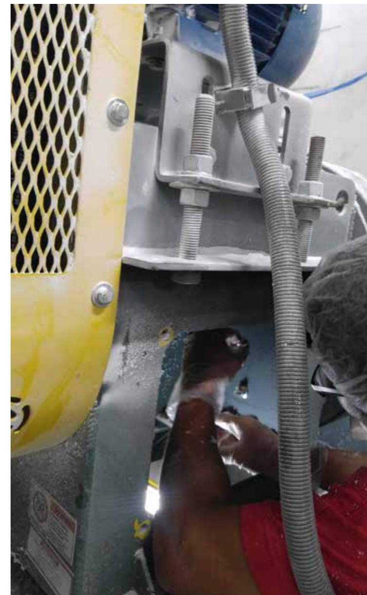
Direct contact with a running motor system with restricted access posed a hazardous risk
